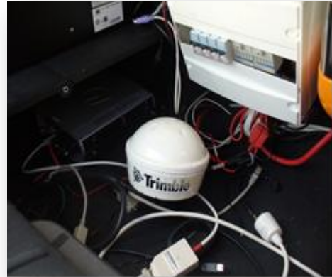
Antenne GPS Trimble
