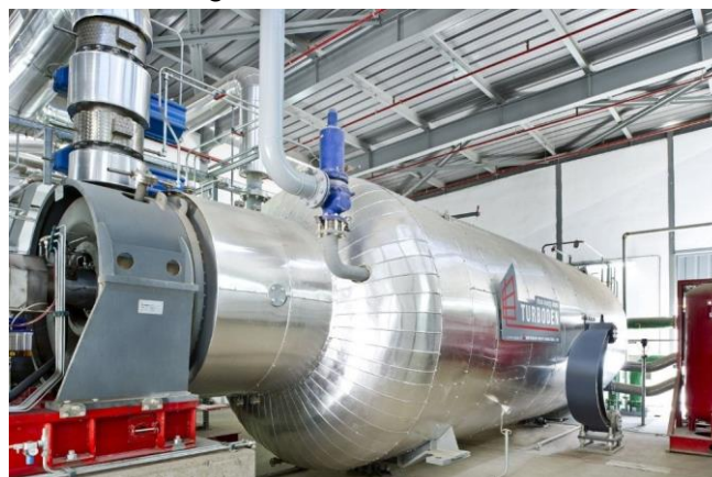
Figure 7 : ORC power plant by Turboden
